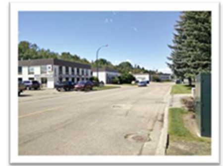
Missing sidewalks along 45 St
